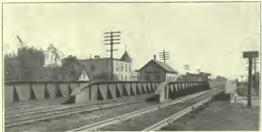
FIG. 272. BRIDGES. Through plate-girder bridge of the Chicago & North Western Railway over street crossing at Avondale Station.
